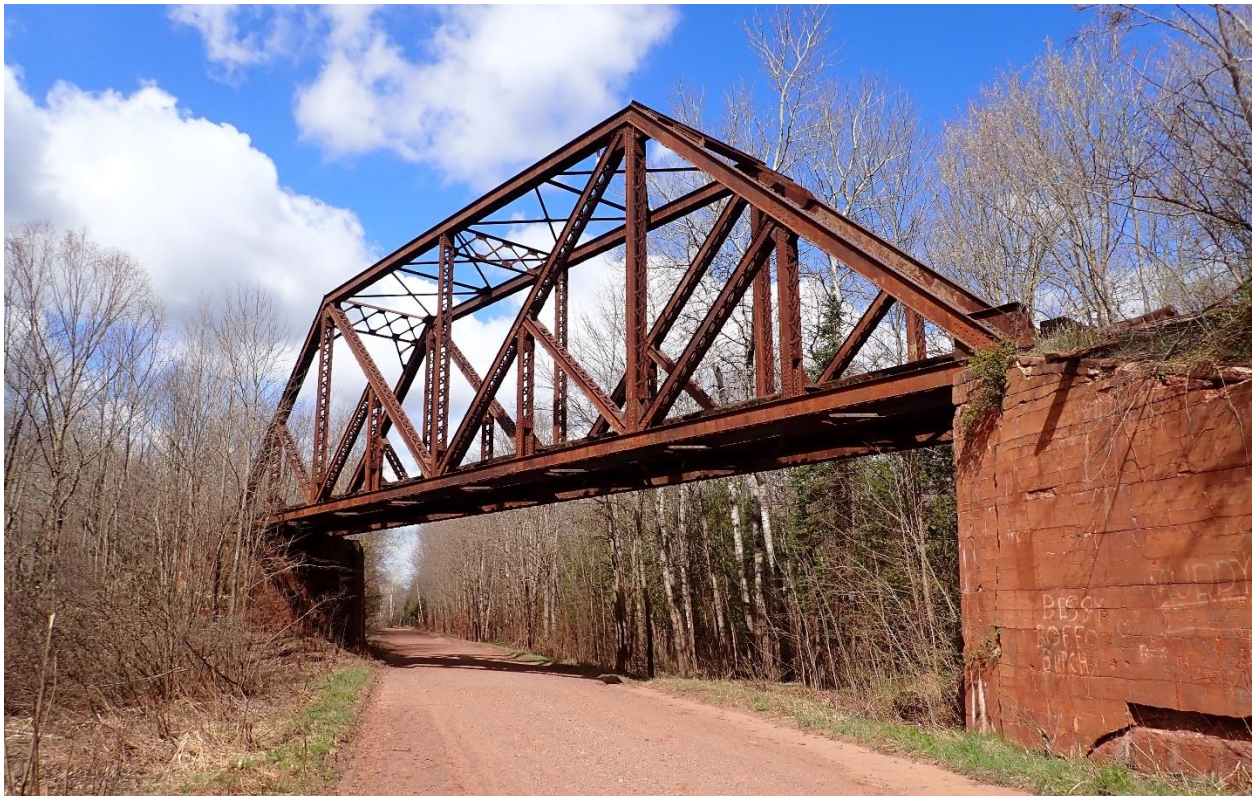
Caption: The Hurley Overpass West bridge would become public property if ICORE and the City of Hurley are successful in completing the land purchase from CN. A paved trail would be built across the bridge, connecting to the existing Iron Belle Trail.
